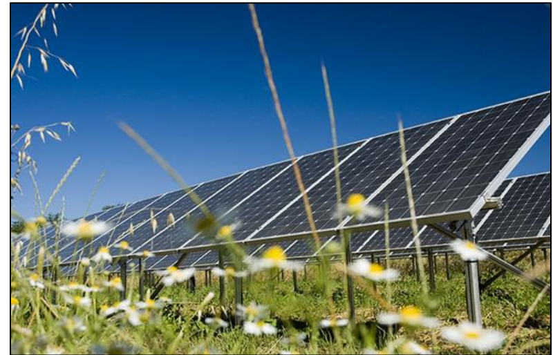
Figure 4.1 Image of ground mounted PV panels
